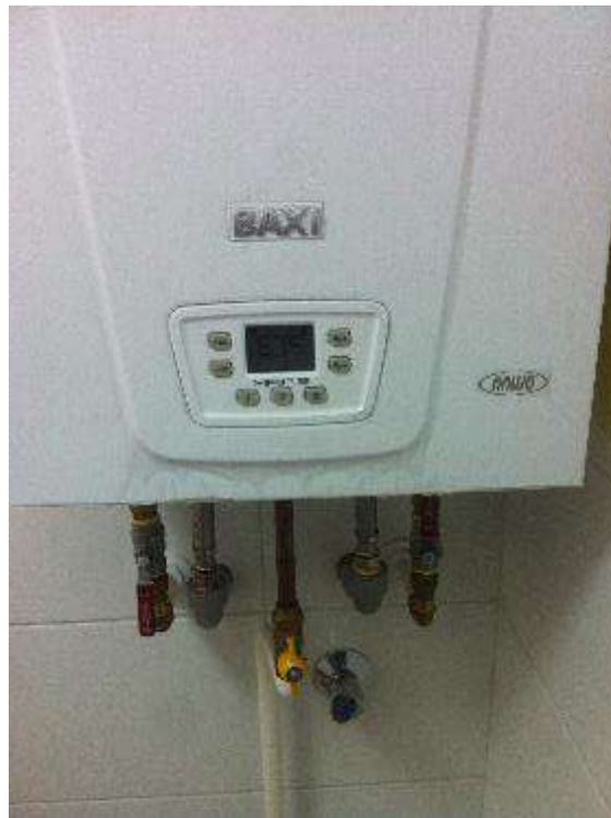
Panel de control.
